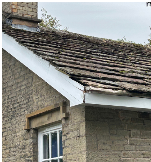
Damage to school building roof
